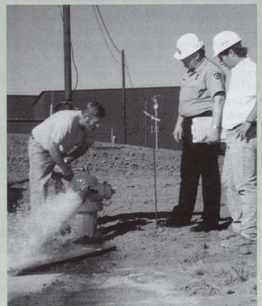
Delhi Charter Township Fire Inspector Craig Whitford (center) checks hydrant pressure at a construction site in Ingham County. On-site inspections prior to occupancy help developers comply with township building and fire codes.
