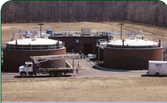
Delhi Charter Township (Ingham Co.) recently received national recognition for developing the state's first integrated biomass-to-energy digester system.
