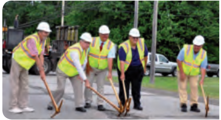
(From left) Erie Township Supervisor Bill Frey, Bedford Township Supervisor Greg Stewart, Rep. Dale Zorn (R-Ida Twp.), Monroe County Road Commission Chair Bob Stammer, and Whiteford Township Supervisor Walter Ruhl held pick axes for the official groundbreaking to reconstruct County Road 151.
